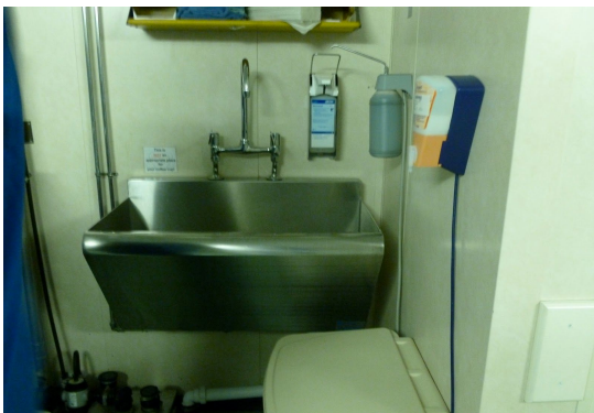
Figure 4.5: Scrub sink in operating room in Guinea. Photo CC BY-SA 4.0 Lifebox
